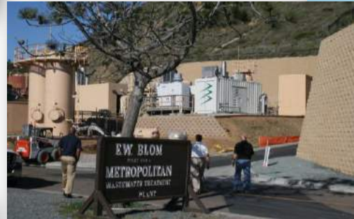
0.3 MW at Point Loma WWTP and Biogas Purification System
