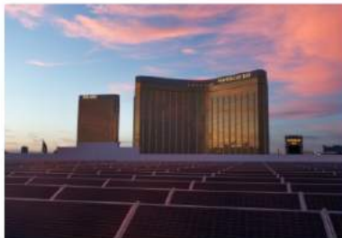
Photo Credit: NRG Energy
